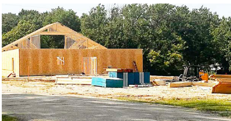
THE ANDERSON COUNTY REVIEW 10-16-2025 / COLONY MARSHAL'S OFFICE Destroyed by arson last December, the new Colony Community Church has been under construction since earlier this year.
