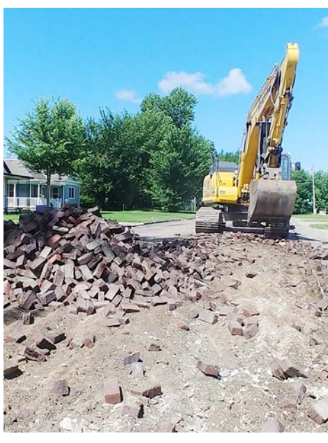
Street refurbishment on 3rd Avenue in Garnett last week yielded the original brick street laid in the 1920s.
