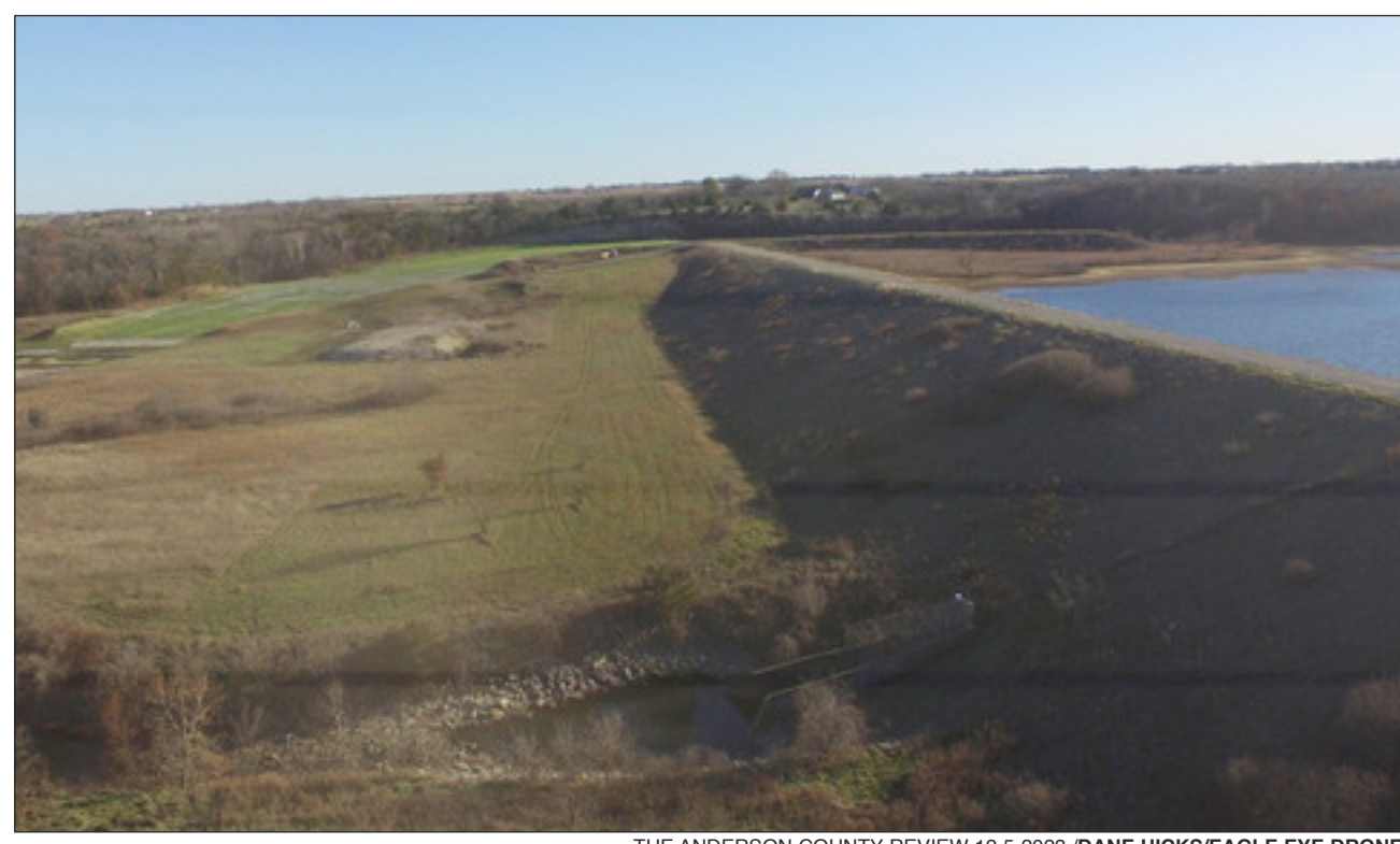
THE ANDERSON COUNTY REVIEW 12-5-2023 /DANE HICKS/EAGLE EYE DRONE An aerial photo shows the recently completed spillway work at the far end of the dam at Cedar Valley Reservoir. The spillway was damaged by torrential rains in 2019, and prior to that was repaired in 2008 after floods in 2007. The base of the structure was rebuilt and shored up to handle advanced water flow. The city received assistance and funding for the project from FEMA.
