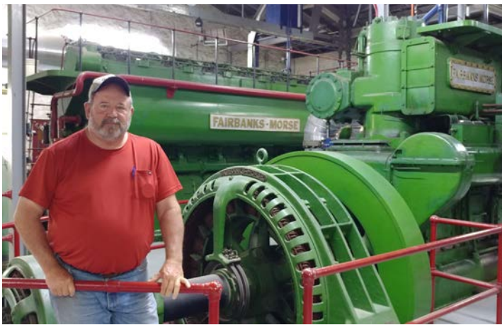
Recent city electric plant retiree Bob Mills poses with one of Garnett's vintage diesel electric generators at the Crystal Lake Power Plant last year.
