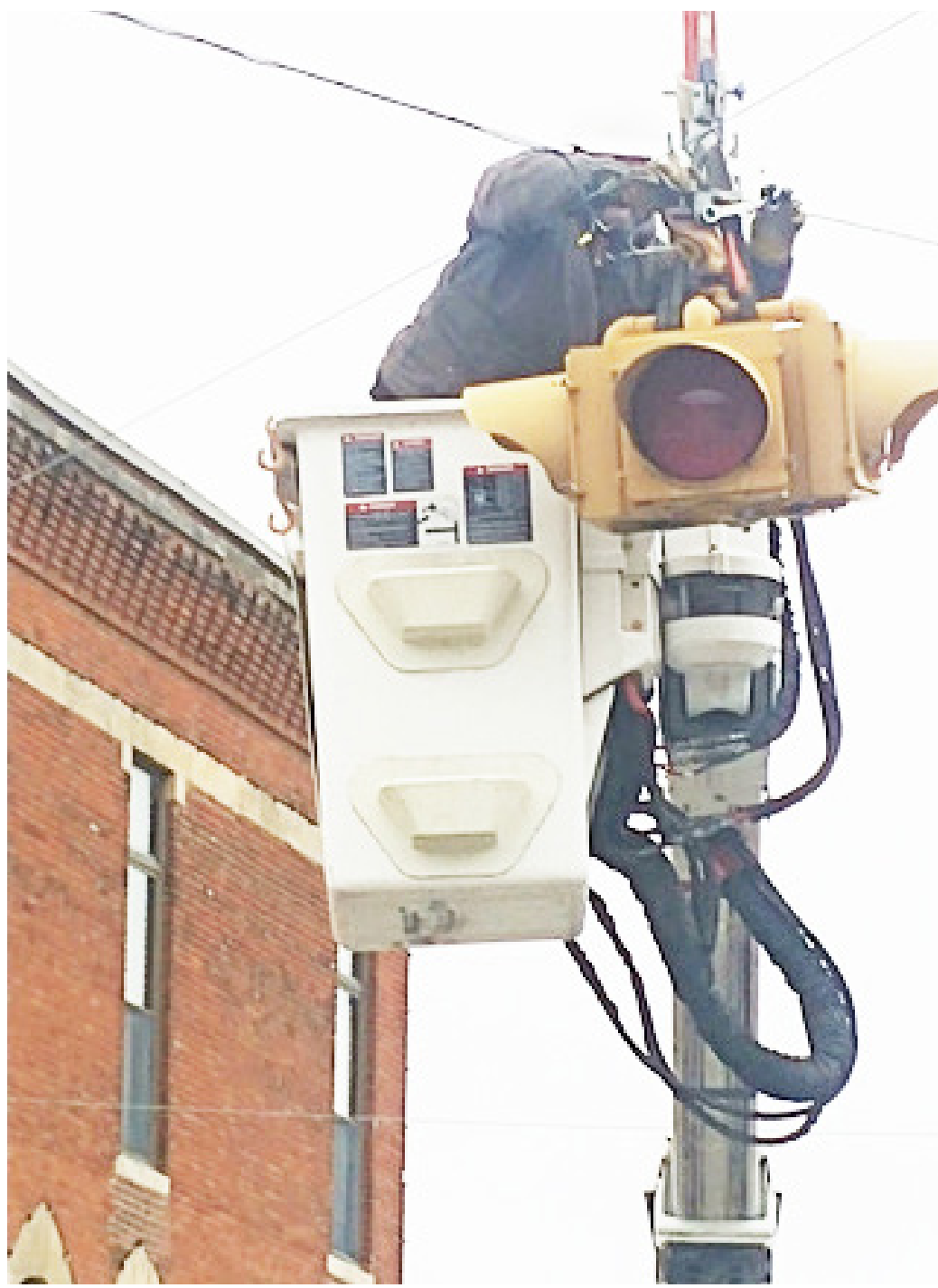
Garnett electric lineman Andy Modlin replaces bulbs in the city's traffic light at Fourth & Maple last week. He got help on the ground from city employee Austin Edens.
