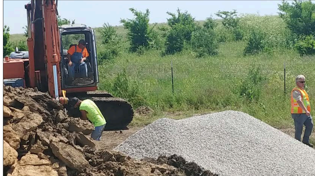
Work crews excavate an area on the right of way of U.S. Highway 59/169 at the project site south of Garnett recently.
