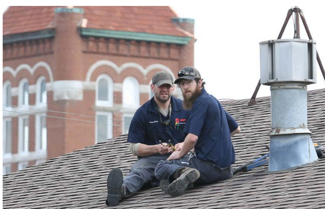
THE ANDERSON COUNTY REVIEW 4-7-2020 / DANE HICKS Kyle Griffeth and Trustin Hays got in some outdoor work on the roof of Farmers Bank in Garnett last week, with a great view of the Anderson County Courthouse.
