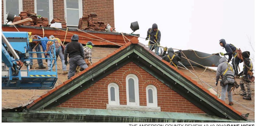
THE ANDERSON COUNTY REVIEW 12-19-2019/DANE HICKS Workmen with Kansas City, Mo.'s, Fidler on the Roof roofing company braved high winds and chilly temps last week to start the re-roofing of the Anderson County Courthouse.
