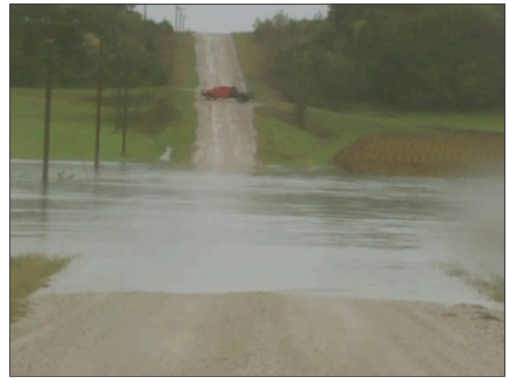
THE ANDERSON COUNTY REVIEW 10-9-2018 / Photo Submitted Road near 2300 and Meade Rd. is impassable and traffic is blocked due to flood waters completely overtaking it on Monday morning.
