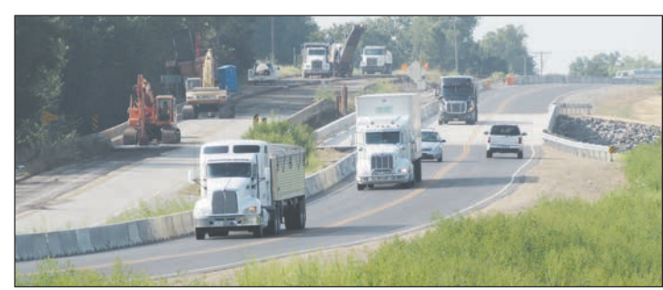
A new bridge over the Pottawatomie Creek was opened in August after nearly a year of construction. The bridge replaced a 58-year-old bridge, seen at left.
