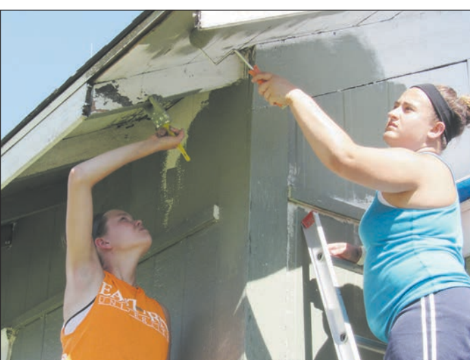
Katie Humphrey and Chelsea Gray, both of Pennsylvania, paint a house as part of GAPP.
