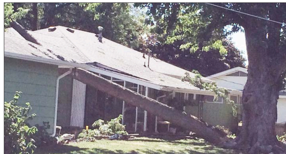
THE ANDERSON COUNTY REVIEW 9-15-2015 / Vickie Moss A large tree branch fell onto an attached garage at this house on Hayes Street during a storm early Friday morning, Sept. 11.
