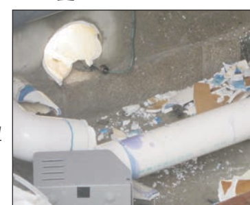
This photo shows some of the damage left by exploding pipes.
