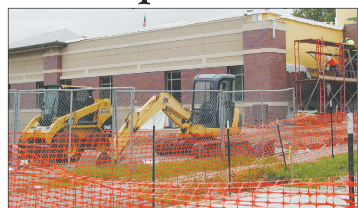
Major construction on the new Anderson County Hospital was completed in 2014. The hospital will open in January.
