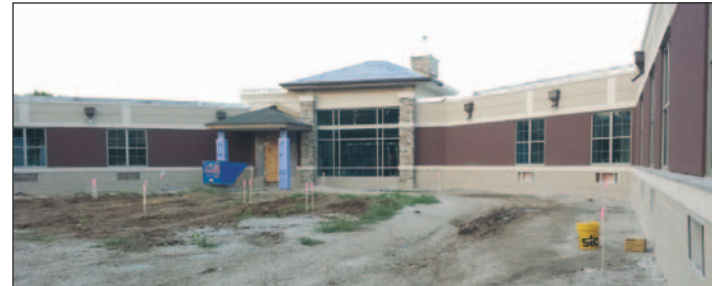
This photo shows the entrance to the new ACH Long Term Care.
