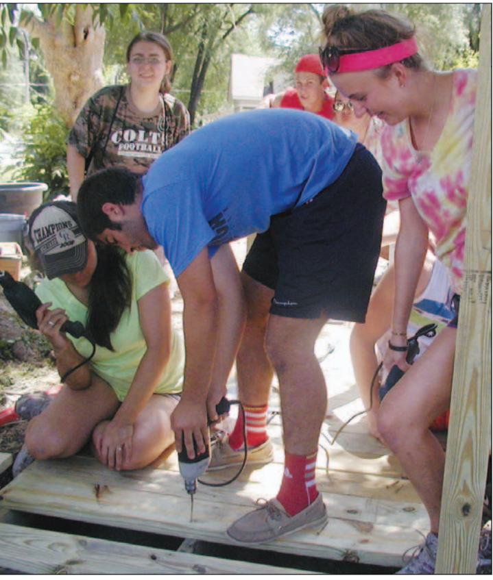
Justin Masri of Indiana screws in a wood plank for a wheelchair ramp at the home of Chris and Diana Bowen on Sixth Avenue in Garnett. Masri and his fellow workers were part of a home repair mission trip that spent a week in June in Anderson County. About 400 volunteers painted houses, repaired porches and built wheelchair ramps.
