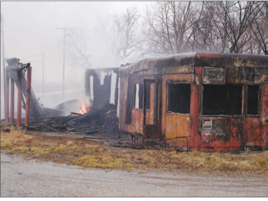
The burned out metal frame of the 1950s diner moved from Thayer to Welda is all that remains of the former Circle B Steakhouse that served Welda and other area residents for many years until it was sold a couple of years ago. Fire officials say the cause of the February fire is not determined, but may have been caused by lightning.
