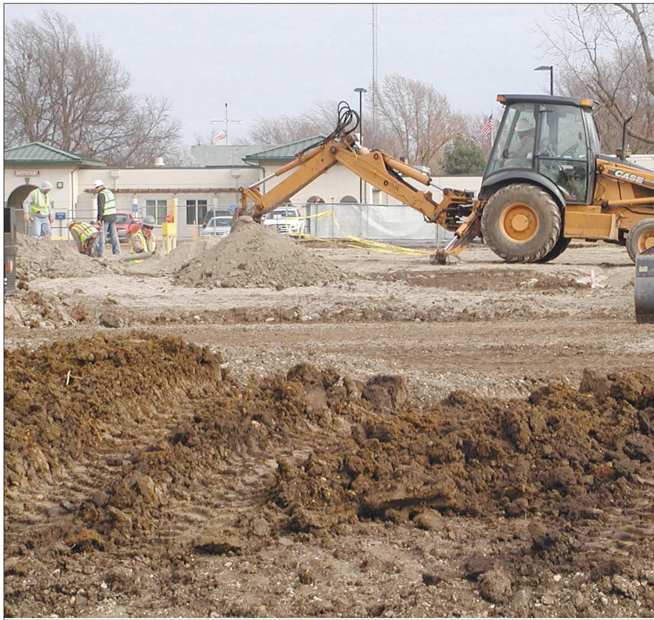
Construction continues at the site of the new Anderson County Hospital Monday, Nov. 25. Crews are continuing to finish dirt and prep work for the site before setting up the structure.
