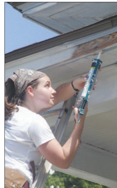
Abby Avery of Indianapolis, Ind., caulks a porch overhang at a house on Sixth Avenue in Garnett.
