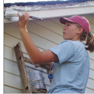
Sam Luehr of Nebraska paints part of a garage at a house on East Fourth Avenue in Garnett.
