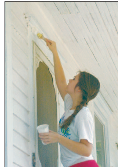
Mackenzie Foulks of Indiana paints a door at a house on Sixth Avenue
