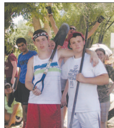
Eric Vergon and Riley Behney, both of Indianapolis, pause while working on a wheelchair ramp on Sixth Avenue in Garnett.
