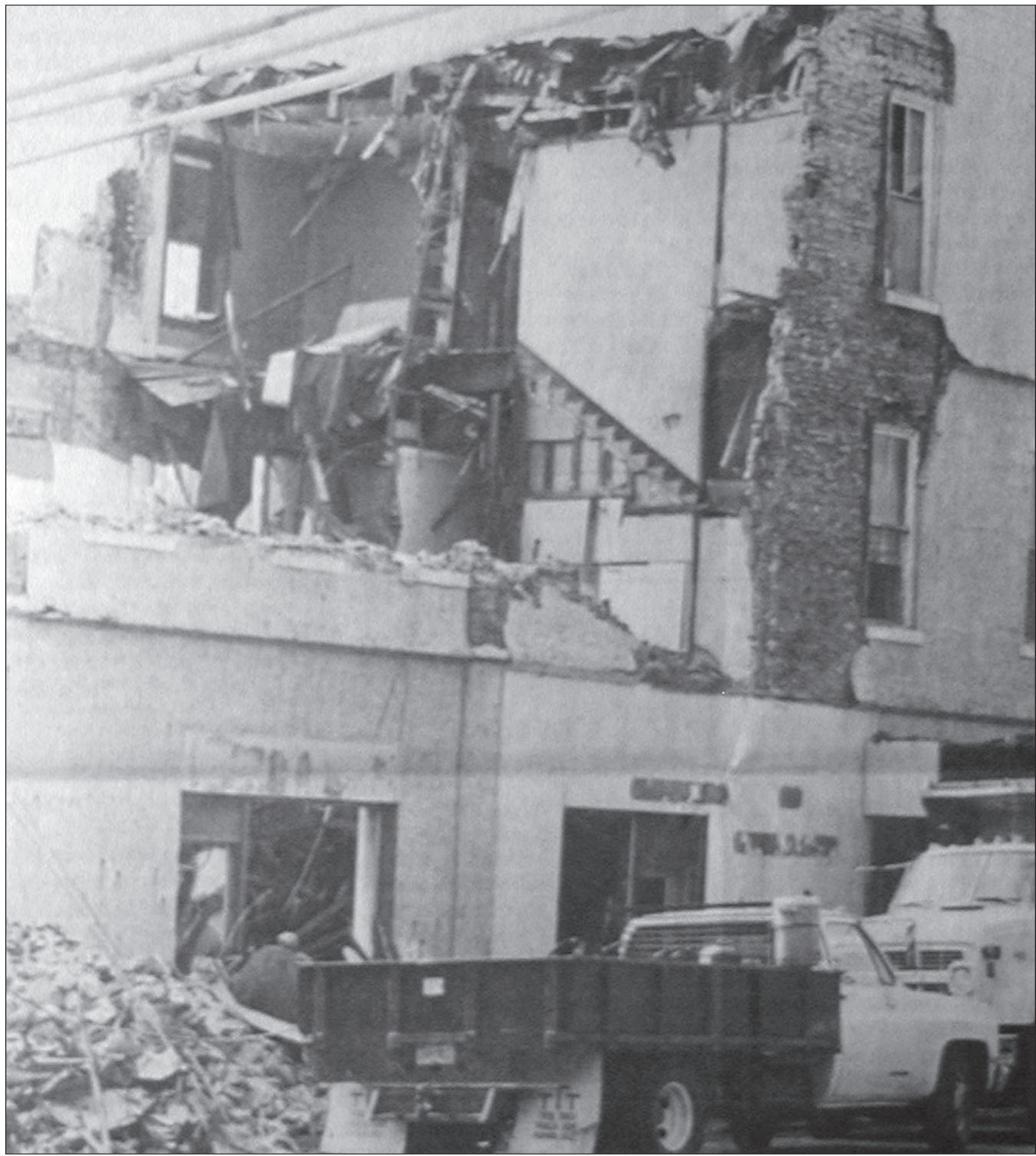
Above, demolition of the Hotel Richart was started in earnest. After two days of work, the demolition crew had removed the back portion of the large structure. The hotel sat at the corner of Fourth Avenue and Oak Street in Garnett.
