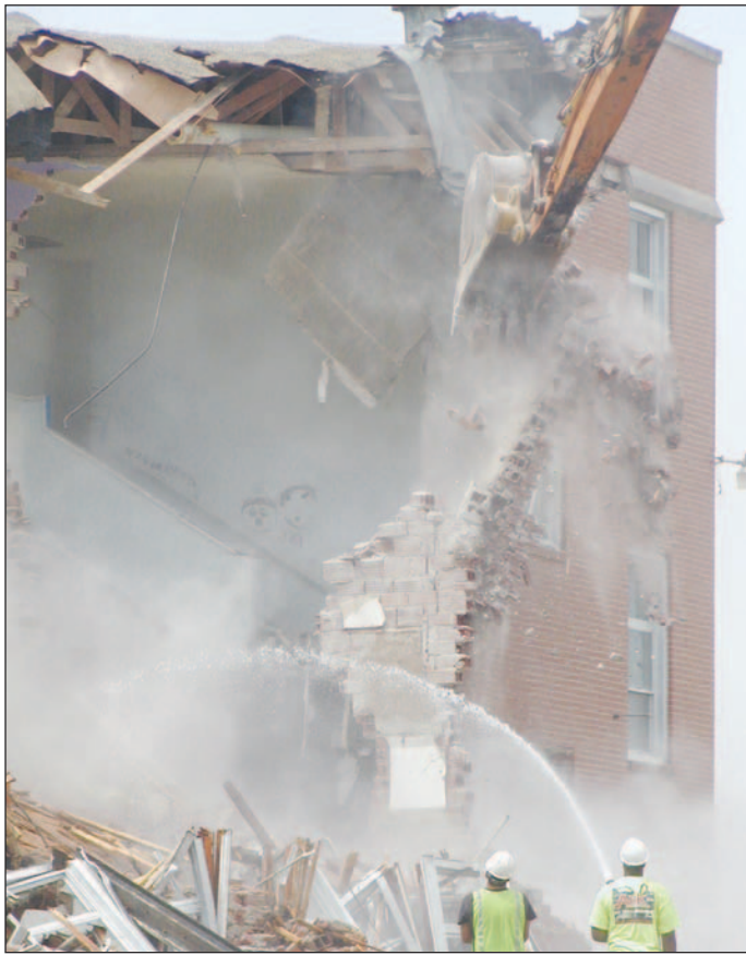
The former Garnett High School/Garnett Elementary Center was demolished in August when a new school opened.
