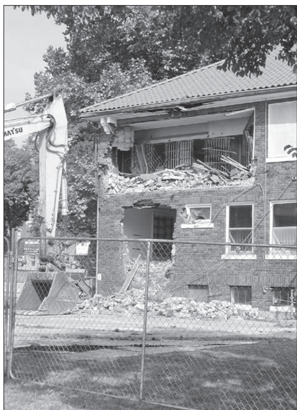
Demolition of the Anderson County Jail barely got underway in the fall when workers discovered what they believed was additional asbestos in the jail's wall linings.
