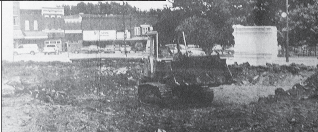
Construction crews clear the way for the new annex building on the west side of the downtown square. It was the first time in more than 20 years that the land was used after fire destroyed buildings on the site.
